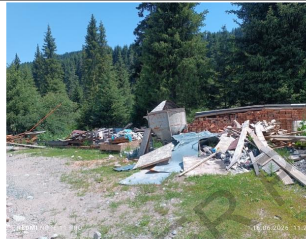
Photo 16: Construction material to be cleaned up
