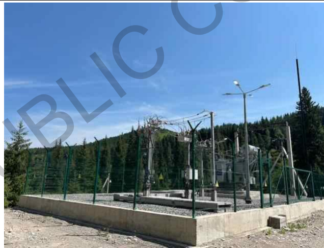
Photo 17: Switchyard next to powerhouse
