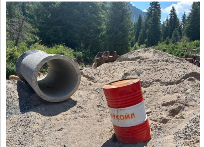
Photo 18: Construction material to be cleaned up
