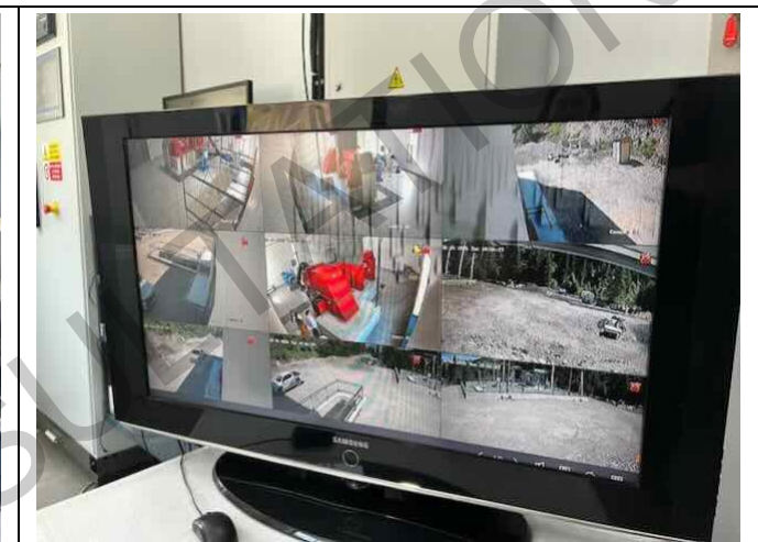
Photo 21: CCTV monitoring from operator's room
